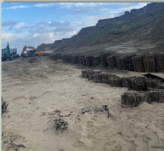
OCTOBER 2020 THE DAMAGE I BEING REAPIRED
