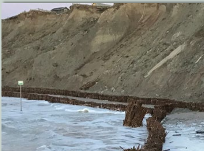
NEWLY ESTABLISHED SYSTEM. 200-300 CM LONG WILLOW FASCINES ARE MOUNTED IN THE BEACH, AND THEY LEVEL WITH 40 CM ABOVE THE TERRAIN.
